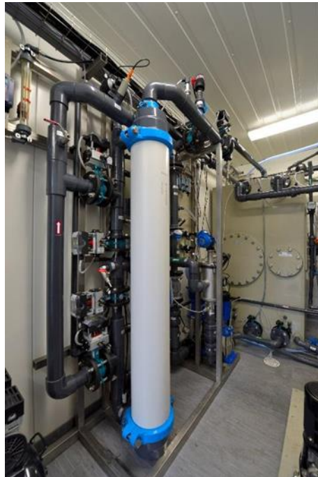
Figure 3. Pilot ultrafiltration unit with one UF membrane module
