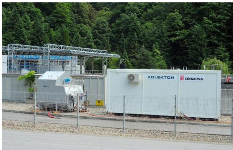
Figure 2. Container with pilot device at WWTP Tremerje
